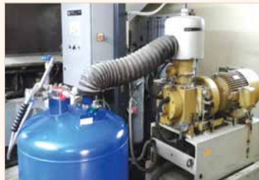
Figure 17: Liquid Nitrogen Facility
