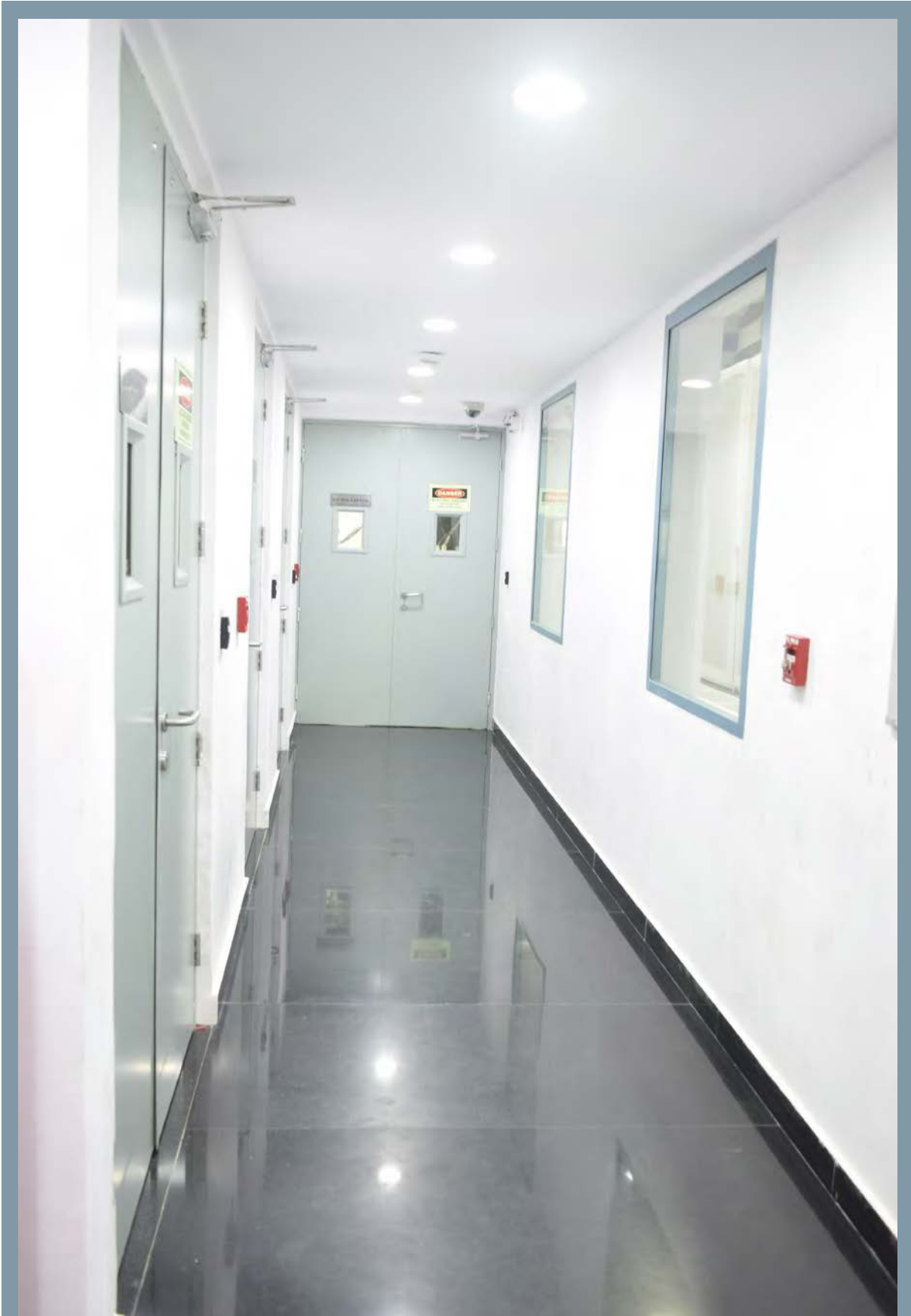
Data Center Corridor of Computer Services Centre
